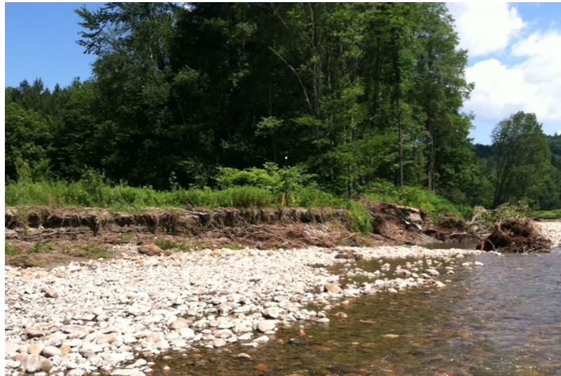
Figure 5. Photo of undercut and eroding bank along Mad River main stem channel, near Lareau Farm Inn in Waitsfield, VT (Site 4 in Figure 5).
